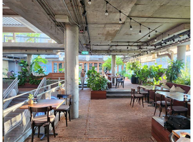
Figure 44 Mechanical ventilation system at the roof.
